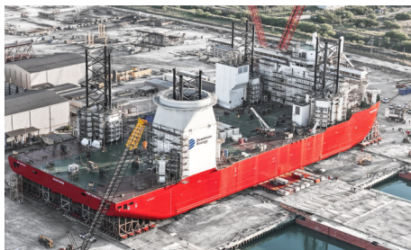
New world record. A total of 880 SCHEUERLE SPMT axle lines moved the “Charybdis” weighing over 23,000 tons.
